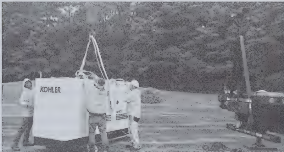
A crane moving in the new generator to the pad at the Safety Complex.
