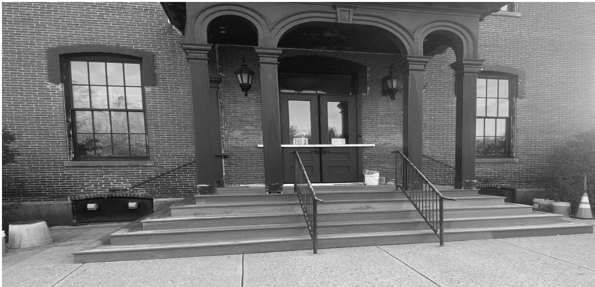
The Historical Main entrance on the west side of the Municipal Complex looks beautiful with its new treads and supports that were rebuilt using a beautiful grain mahogany.
