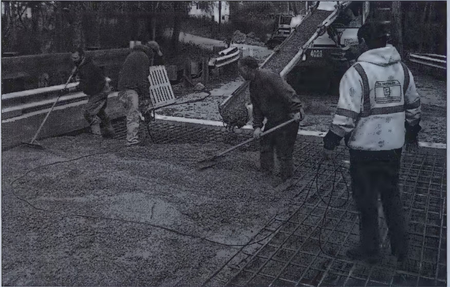
AJ Hartford (right) oversees pouring of the new deck on the Nute Road Bridge over the Bellamy River.
