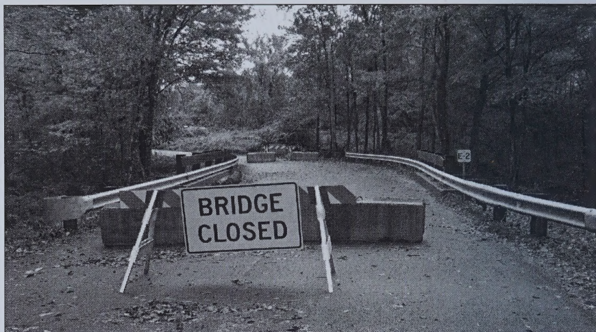
After notification from the State, the Nute Road Bridge over the Bellamy River is temporarily closed while repairs are made.
