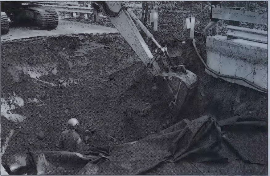
Careful digging prior to pouring new footings at the Nute Road Bridge over the Bellamy River.
