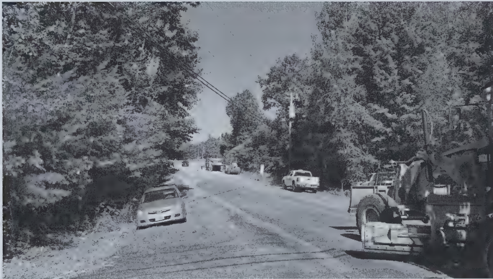
Prep work on Whittier Drive before new pavement 26 July 2016 Photo courtesy of Heidi Carlson
