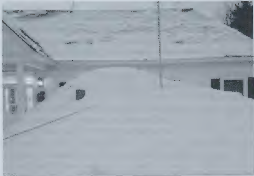
Snow removal from the roof of the Safety Complex in February 2015. Photo Courtesy of Mary Wheaton-Pinder
