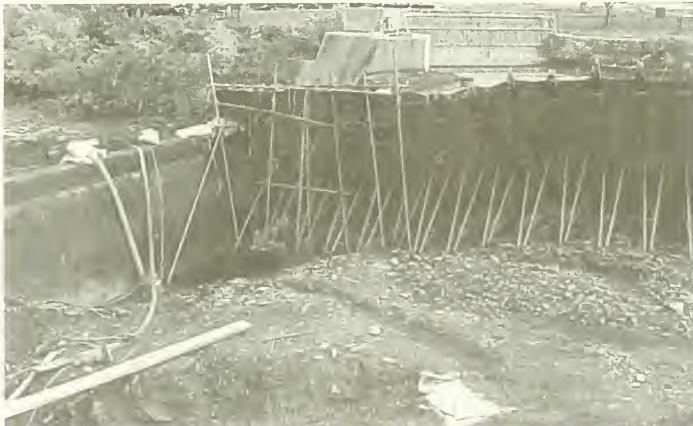
Coffer Dam holding back Exeter River – exposing bottom – during repair to fish ladder – September, 2000
