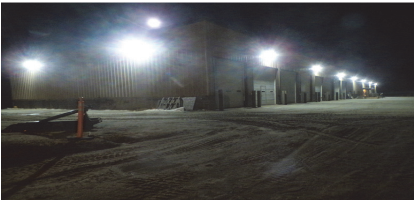
Nine new lights installed on the DPW building. (Light on the roof is the moon.)
