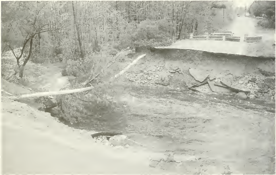
The culvert on Dunklee Road passing over the Bow Bog Brook washed out during the heavy rains and flooding that followed the storm on May 15, 2006. The pipe exposed on the left side is the underground gas line that did not rupture. Once discovered, however, the gas flow was shut off. (Photo by Eric Anderson)
