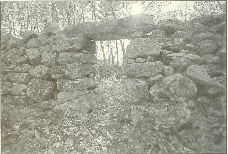
The Town Pound is located on Branch Londonderry Turnpike East. It was built in 1821. The Heritage Commission is working to have some of the stone structure reset to square up and stabilize the wall surfaces for the next 100 years. (Photo by Erik Anderson)
