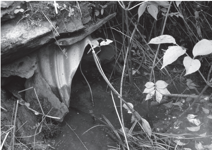
Ageing culvert on Hayes Rd.
