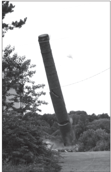
The Elliot and Son's greenhouse chimney was demolished on July 7, 2016. J. Davis
