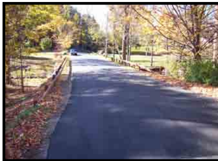
WRIGHT ROAD CULVERT REPLACEMENT AND ROAD WORK PHOTOS: NORTHERN NEW ENGLAND FIELD SERVICES, LLC
