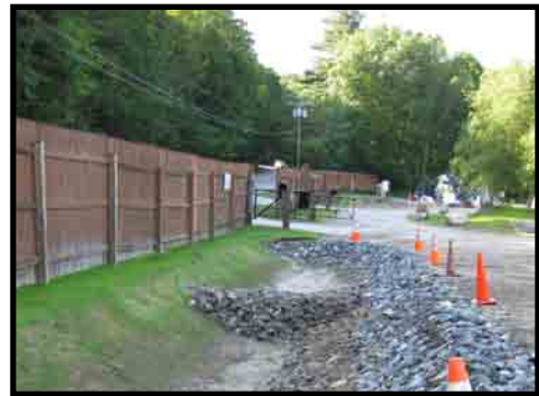
STORMWATER MANAGEMENT AREA AT THE TRANSFER STATION PHOTO: CATHY HOFFMAN
