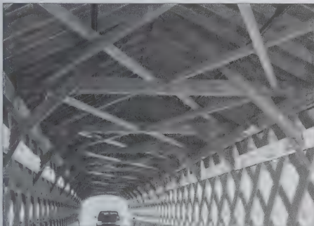
Sprinkler piping as seen from bridge roadway
