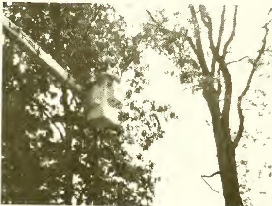
Repairs from wind damage
