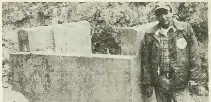
Rick Parker of Manchester Redimix donated his time, truck, and materials for a bridge foundation for the Heritage Trail.
