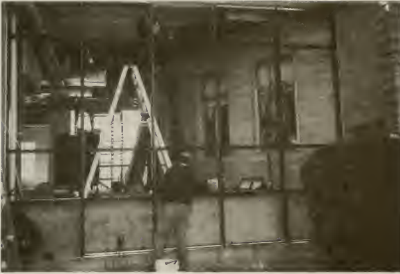
Old meets new. Original building and the beginning of ones of the glass curtain walls.
