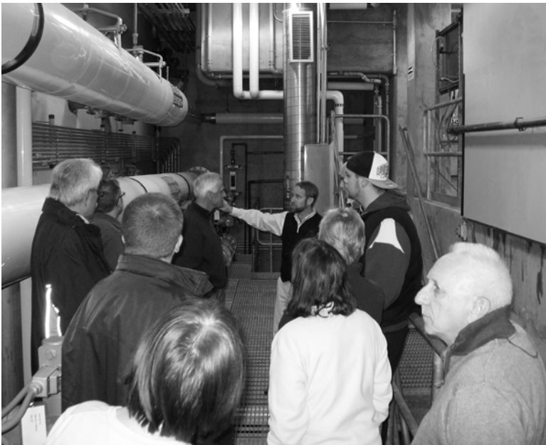
Peter Rice (center back), from Portsmouth, explains aspects of the water treatment plant's filtration process. E. Fiegenbaum
