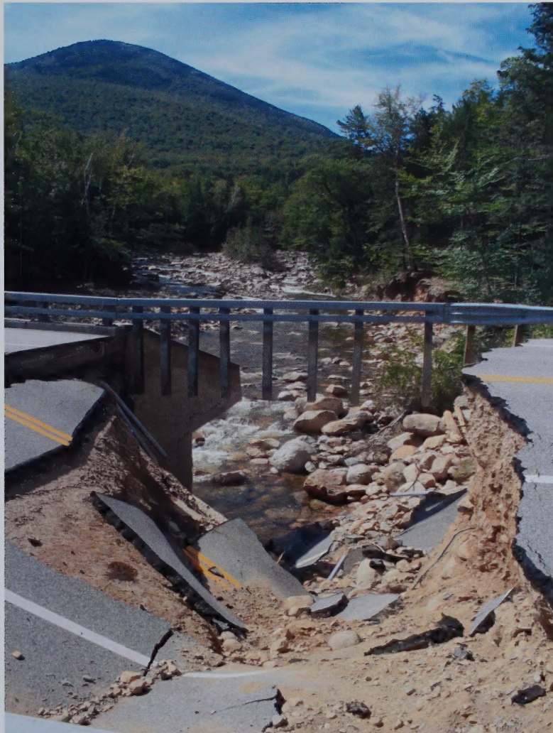
Bridge Out, US Route 302, Sawyer River
