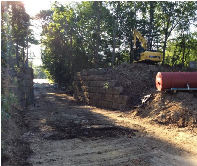
The above photo is the section of roadway between the abutments as we were getting started. (Credit NEFS)
