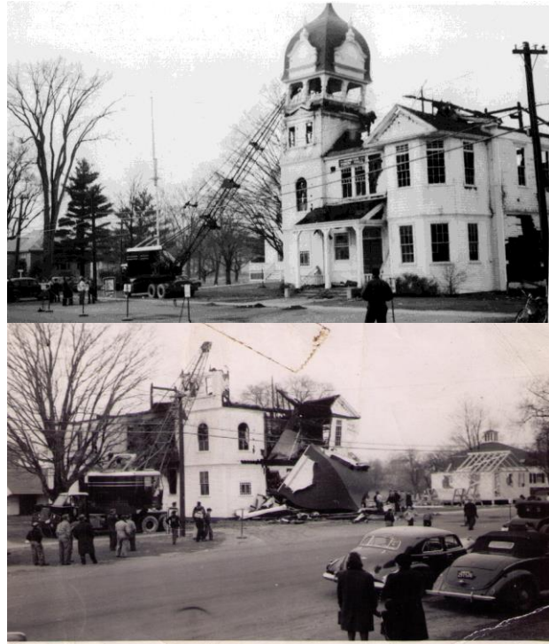
Toppling of the Tower. "Temporary" structure to the right of the Building.
