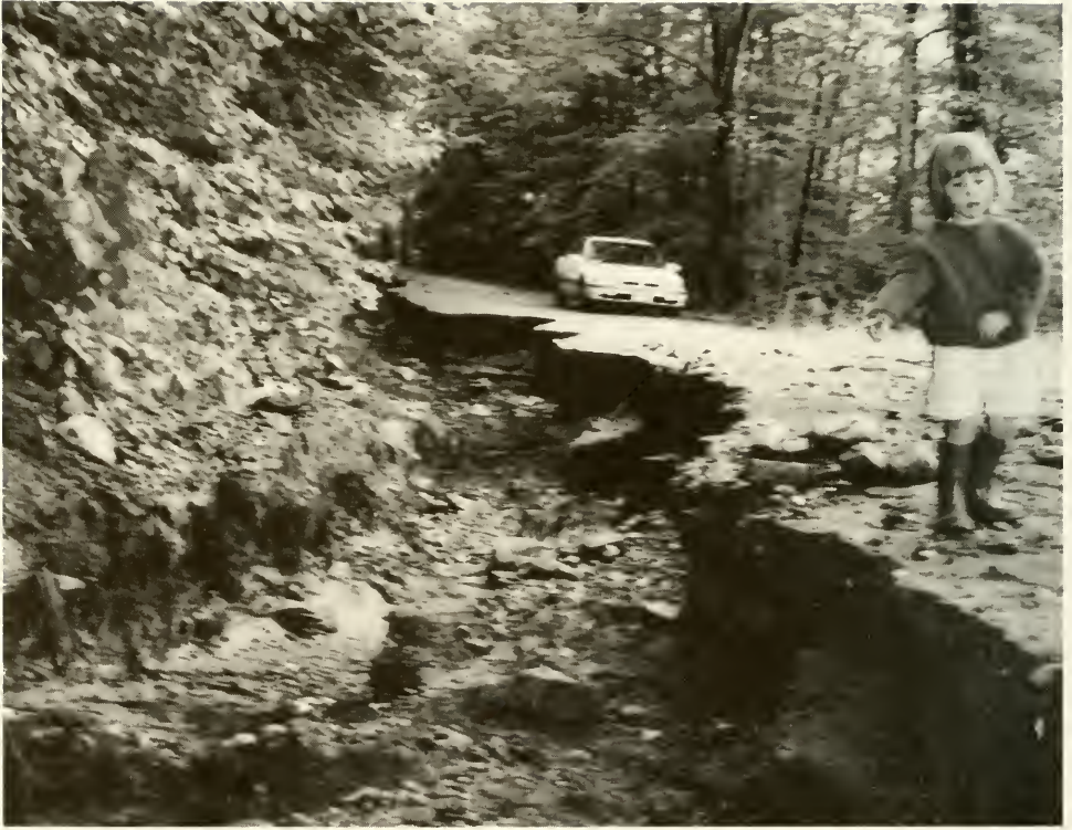
Megan Thibault checking out the damage caused by heavy rains on Tandy Brook Road in the Spring of 1998
