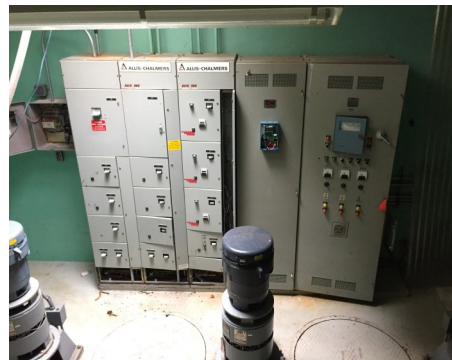
Main control panel in the dry well of the pump station after the water was pumped out. Our pump motors are in the foreground. Everything you see here was completely submerged.
