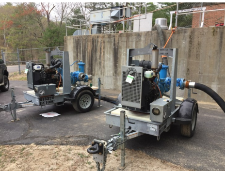
Rented generator pumps pumping wastewater up to the treatment plant
