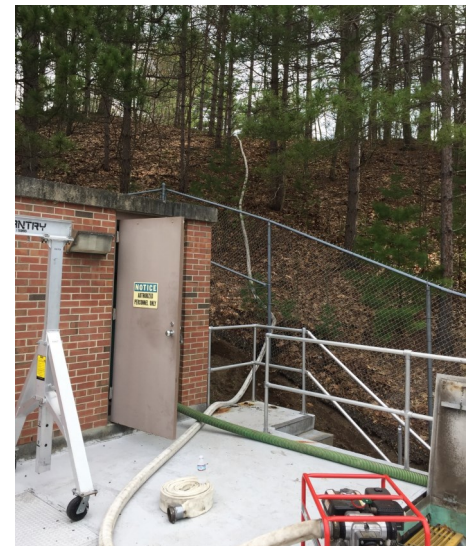
One of our pumps pumping wastewater up to the treatment plant
