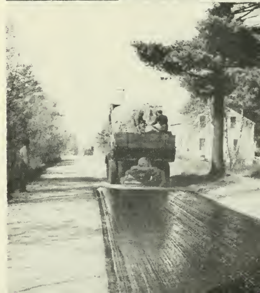
(Top) Quantity production of road-patch material at the city sand pit (Center) A grader and tar truck team-up to re-surface a country road (Right) A mechanical spreading unit sanding newly applied tar
