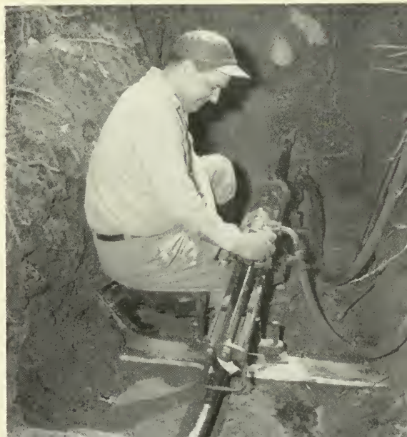
A waterworks employee operates the department's newly acquired flexible service cleaner to ream out a clogged house connection
