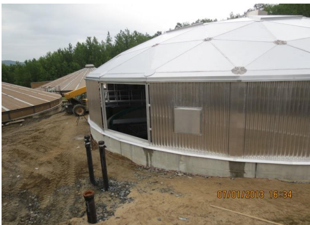
The New Secondary Clarifier with covering dome structure
