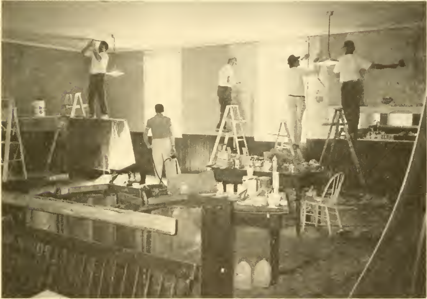
Old Town Hall Project: Rotarians scrape, patch, and paint the ceiling, scrape off the old wallpaper and prepare the walls for new paper, scrape and prepare the trim for painting, and ready the floor for resurfacing. Rotarians have already scraped and painted the kitchen and toilet areas as well as installed new lighting. This community project is ongoing. (Photo by Eric Anderson)
