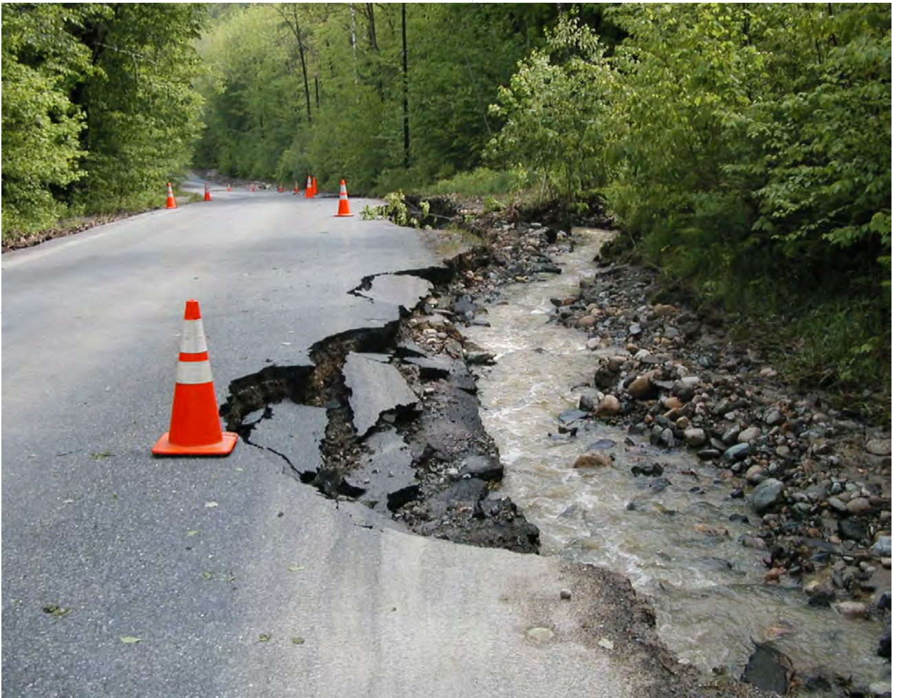
Damage to Slate Ledge Road on May 27, 2011.
