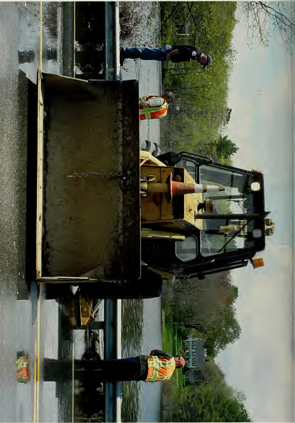
In the aftermath of the flooding in Hampton Falls, Road Agent Richard B. Merrill Sr. lowers the water at Whittier pond by using his backhoe to remove two planks from the Dam. May 2006
