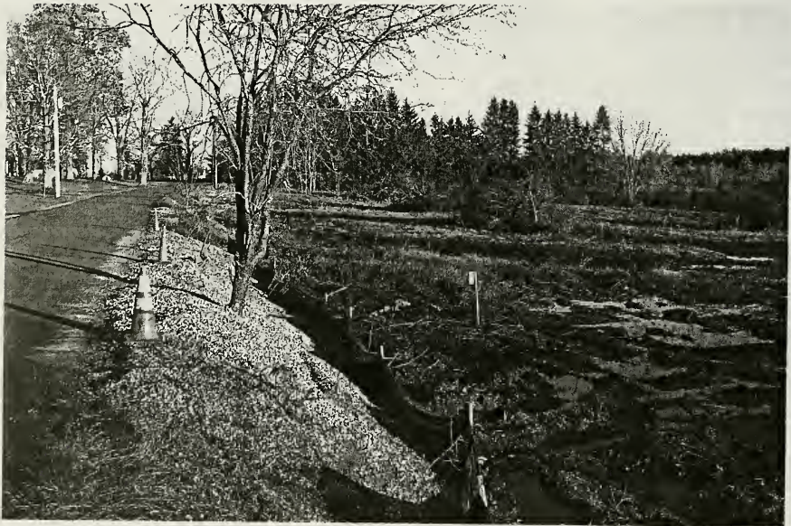
Shoulder on Brown Road that was recently rebuilt by the Road Agent Richard B. Merrill Sr. November 2006
