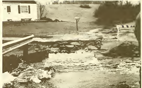
Adams Pond Road Flood Damage
