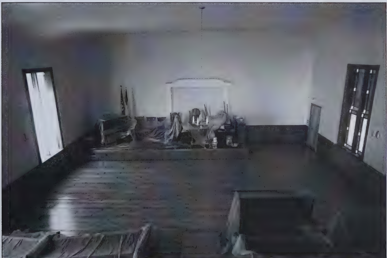
The East Grafton Union Church sanctuary, with its new paint and refinished floor.
