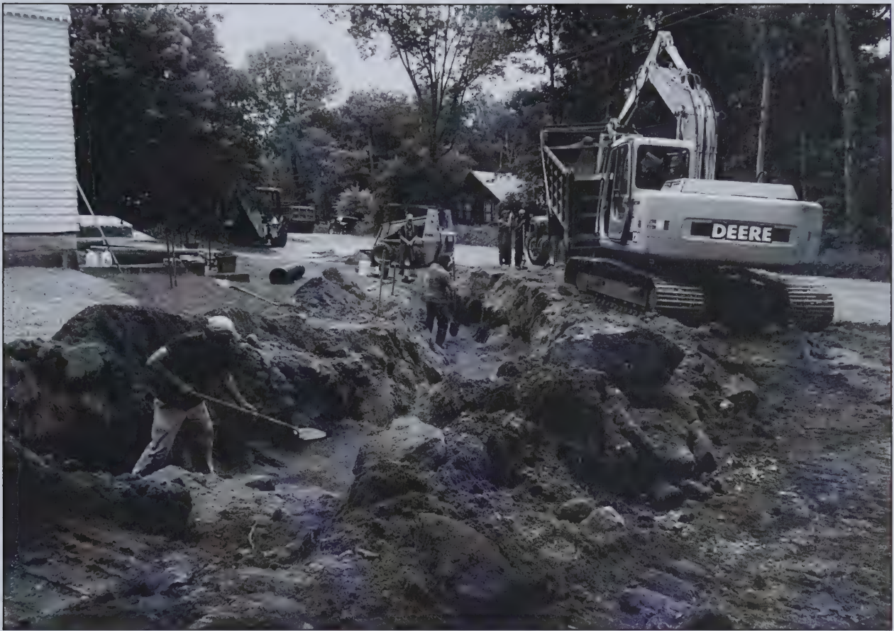
Razor Hill Excavation's crew digs new perimeter drainage at the East Grafton Union Church.
