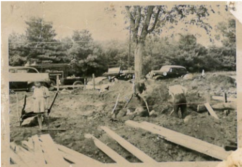
Bottom photo the foundation and starting the west wall. Circa 1946. Courtesy Barrington Firemen's Association collection.
