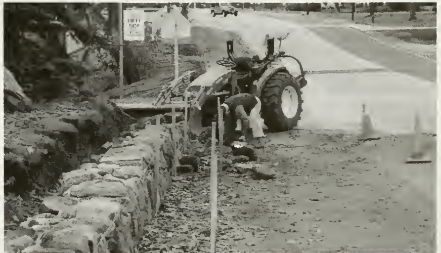
New sidewalk under construction. Chris Norris hard at work at his new "day" job.
