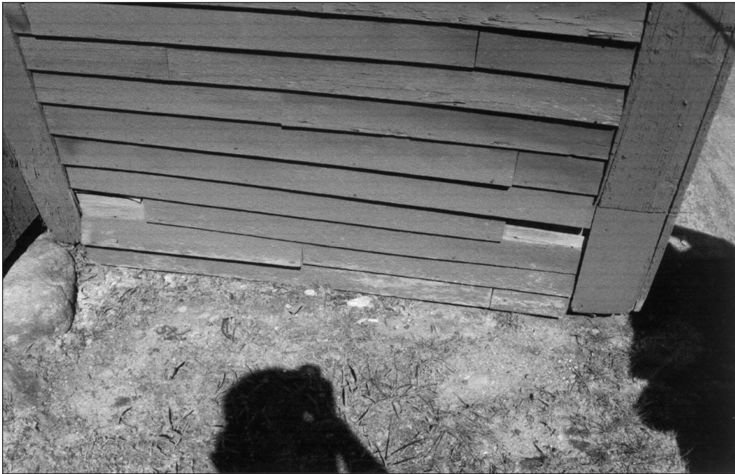
Bottom of entry way - road side - missing and rotten pine clapboards
