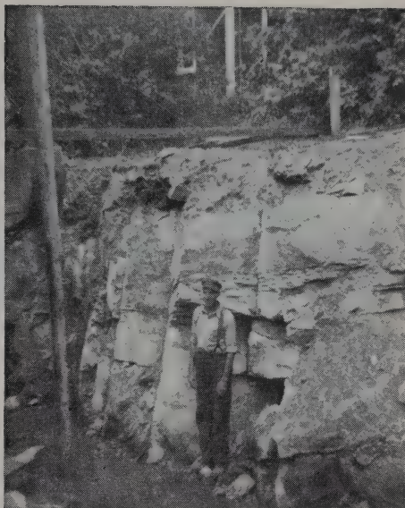
The Rule Street sewer project was like this for a distance of 600 feet, requiring a 12-foot depth of blasting into solid ledge.
