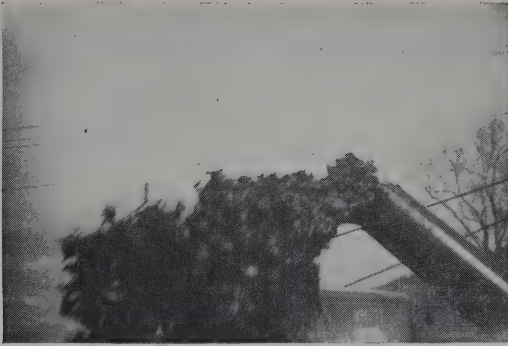
Cleaning the main at Marlboro Street just before "the rabbit" came out.
