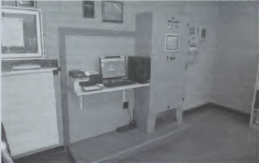
New Operations Control Panel
