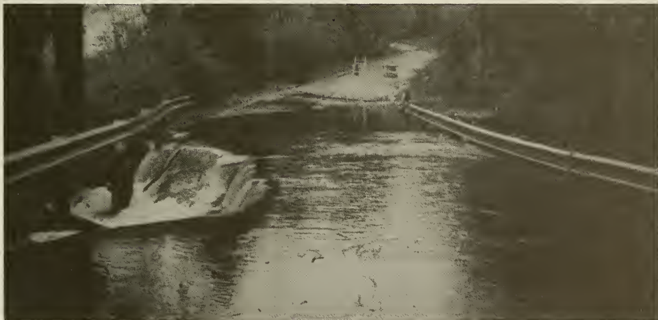
A section of Drinkwater Road culvert at King Street and Town Forest damaged by the flooding on October 21, 1996 photo taken by J. Timothy Samway
