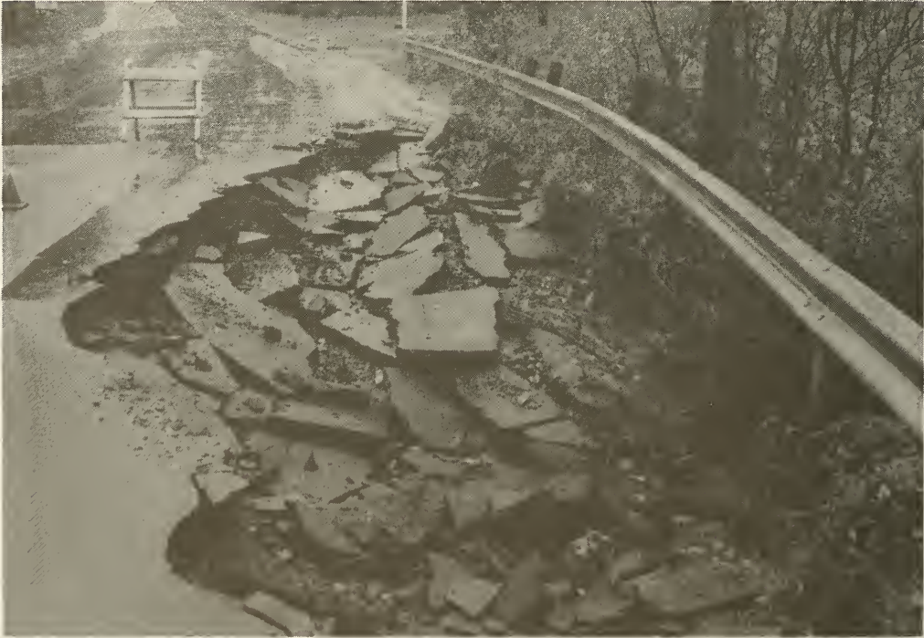
A section of Drinkwater Road near the Bricketts damaged by the flooding of October 20-21, 1996. photo taken by Jack McEachern
