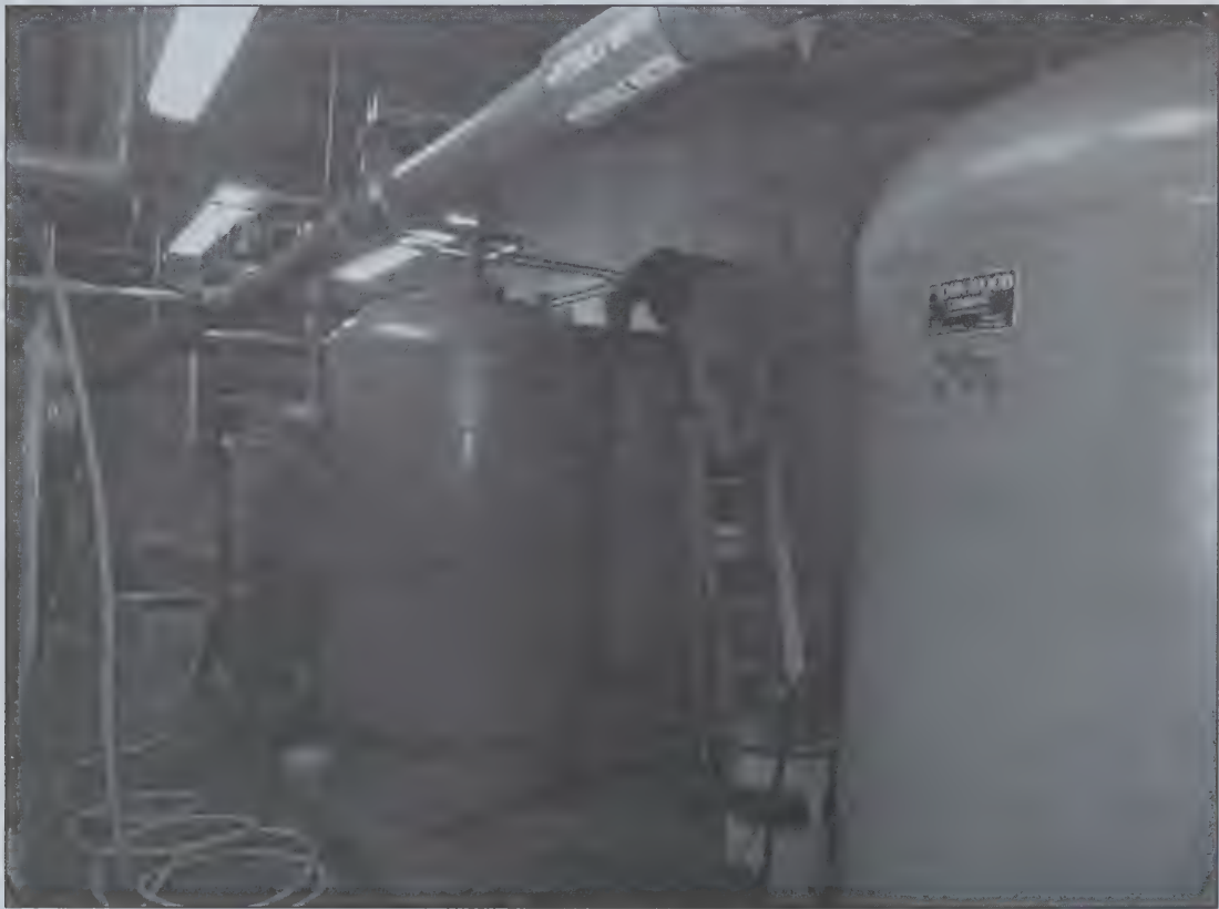
New pressure bladders being installed into hydro pneumatic vessels at the Water Treatment Plant
