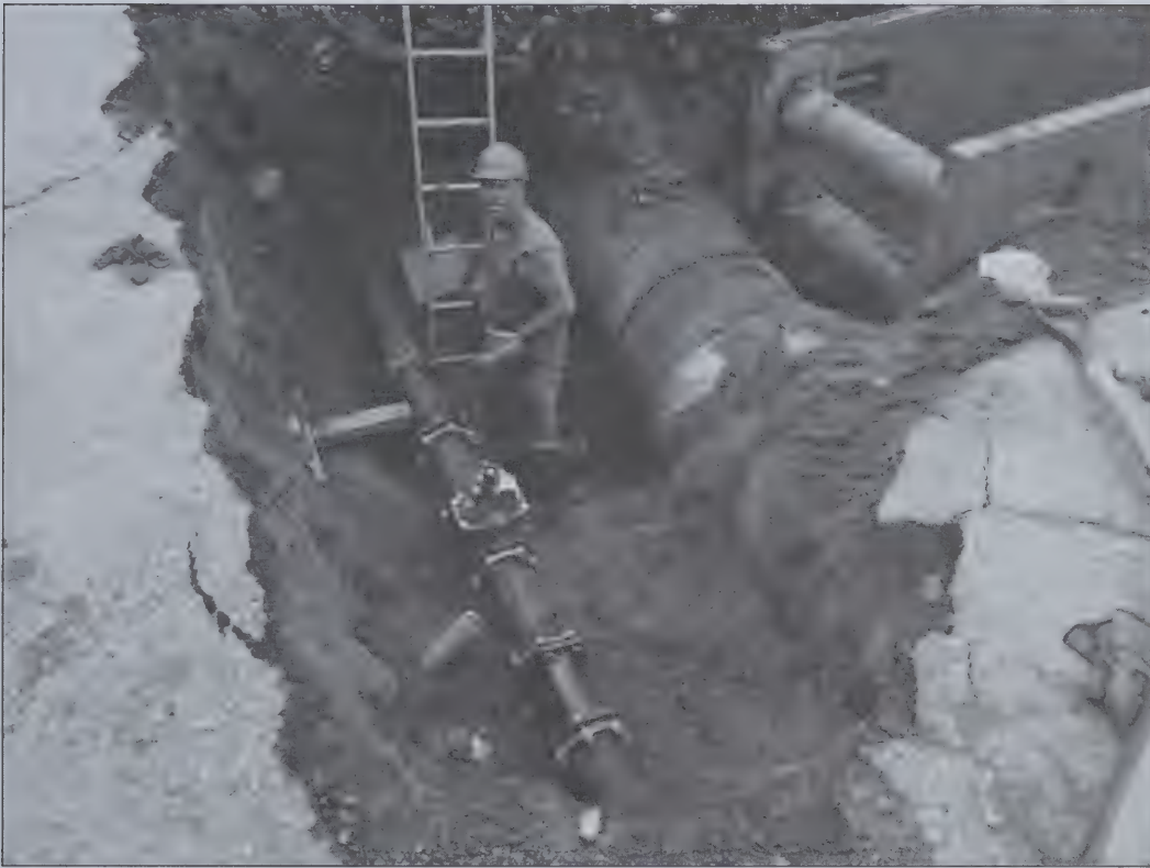
New 6 and 8 inch resilient seat valves installed on the intersection of Willis Place and Alpine Street
