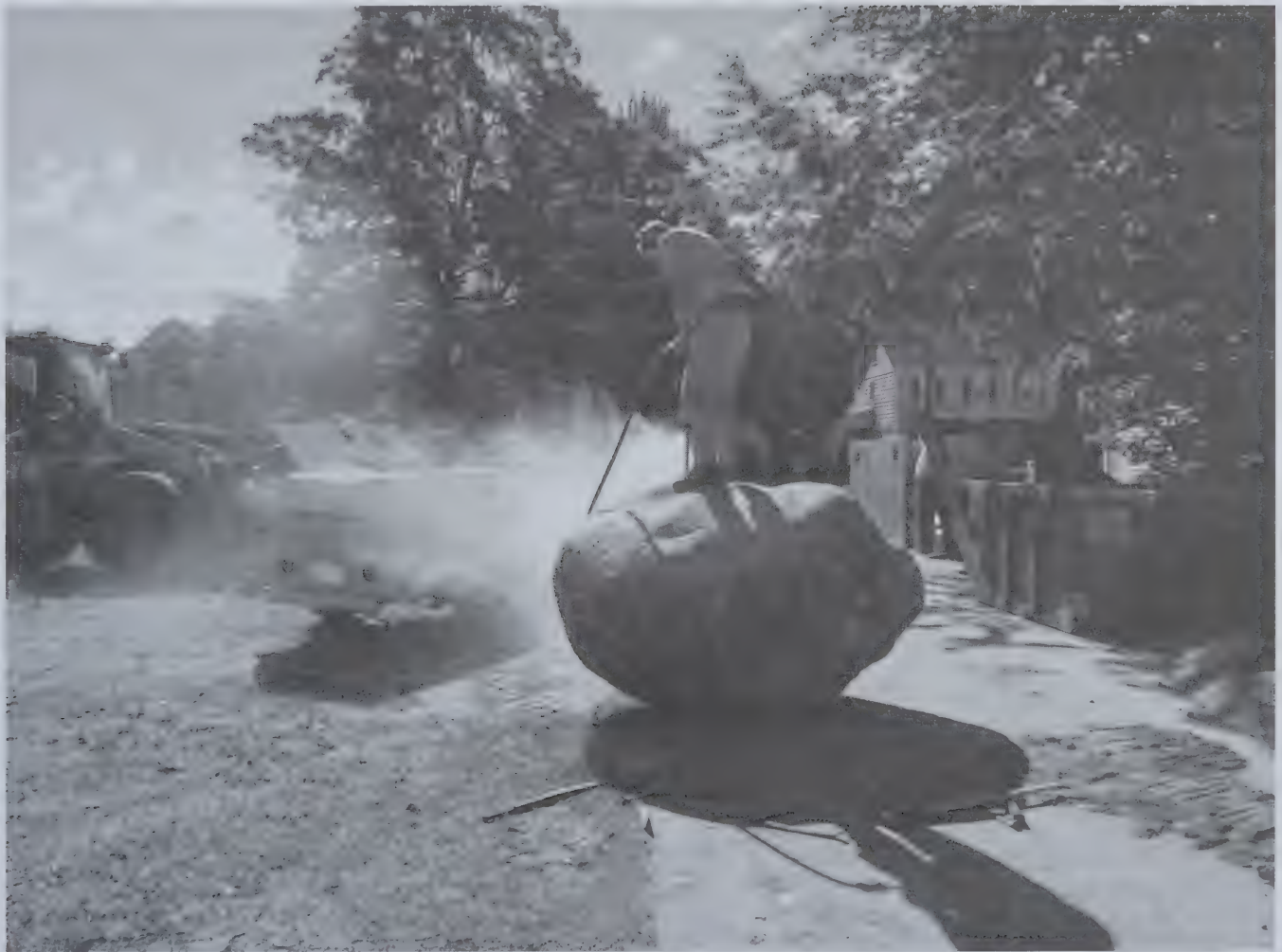
Preparing to split large rock for removal at Willis Place Water and Sewer main replacement project
