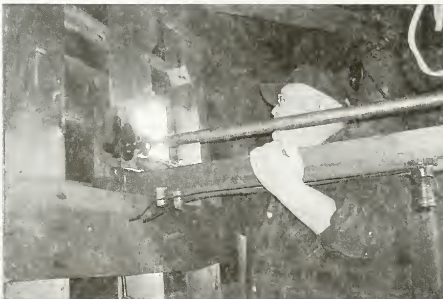
Murray talks with Richie, who is outside on the ladder, through a hole in the north face as he works inside on the northern-extending gear shaft.
