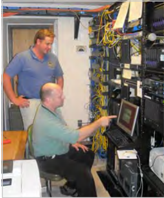
IT Coordinator Alan Brady and Seacoast Computer's Gary Rooney oversee the City Hall server room
