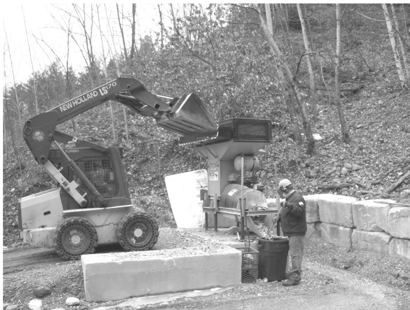
ABOVE: Pete Fernandes(in the skidsteer) and Marc Boisvert crushing glass, saving money on disposal costs and creating a useful aggregate product for our highway department.
