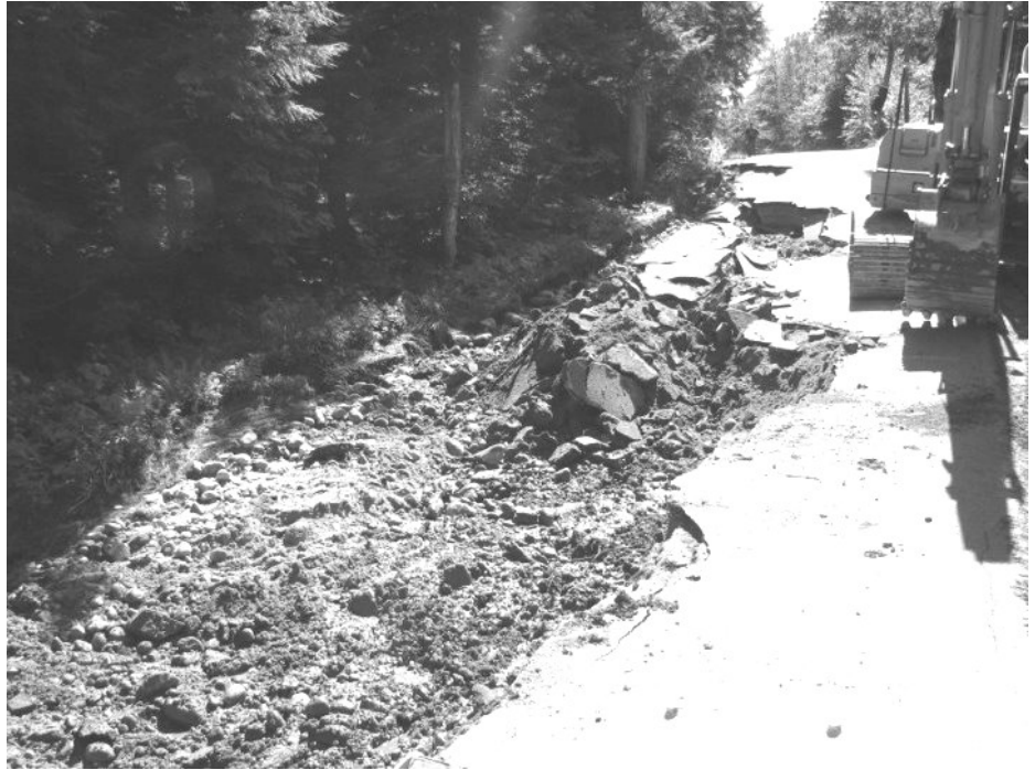
ABOVE: Parts of Craney Hill Road were severely damaged during Hurricane Irene.
