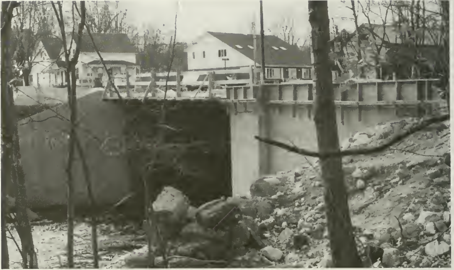
The Cilleyville Road bridge under construction. This photo was taken in the fall of 1996, by Roger Emerson.
