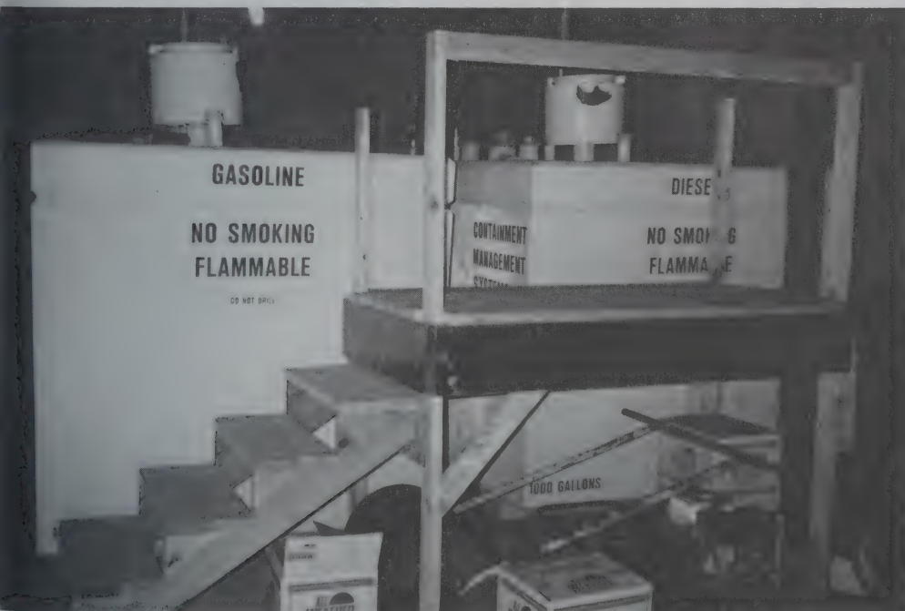
Town fuel tank facility for all town vehicles – gasoline and diesel tanks – located at Incinerator Recycling Facility.
