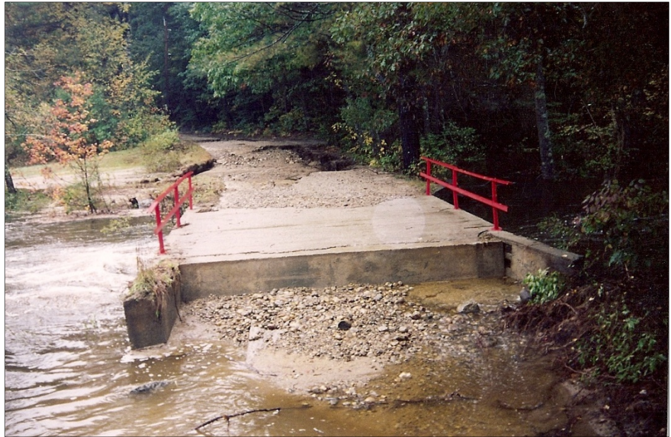
Flood Mother's Day 2005 - Sleeper Road Bridge
