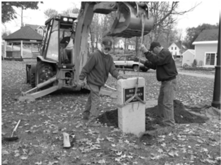
TOP: Marc Boisvert and Pete Fernandes repairing and replacing park benches at the Old Concord Road Soccer Fields. BOTTOM: Selectman Ron Taylor and Assistant Superintendent Pete Fernandes install a new historical marker at Community Park on Main Street.
