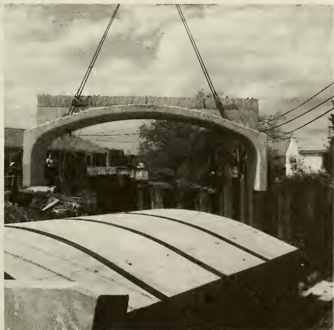
The October, 1996 Storm washed out Eel Creek, causing substantial flooding. Through the efforts of the Town, State agencies and Emmanuel Engineering, the box culvert was replaced with this pre-fabricated concrete bridge.
