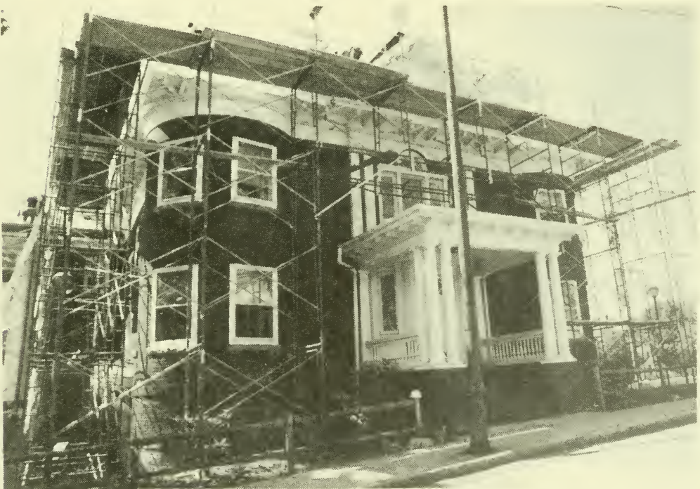
Reroofing and trim painting at Charpentier's (Formerly Saint Martin Rectory and School)
