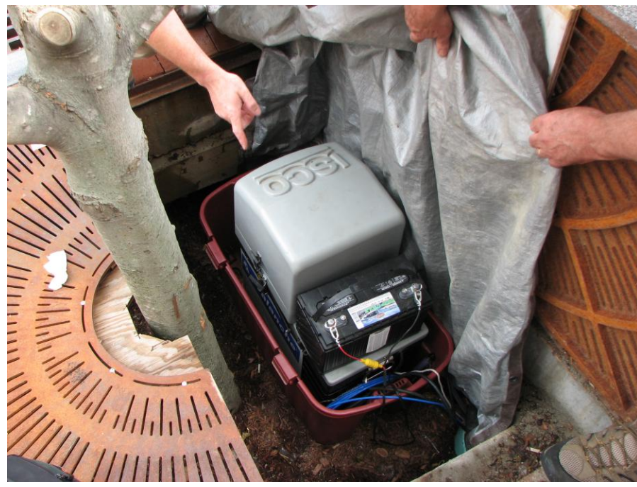
Photo 4: This shows the effluent sampler installed inside the tree box during the monitoring phase. The location is represented by the red dot in figure 1.
