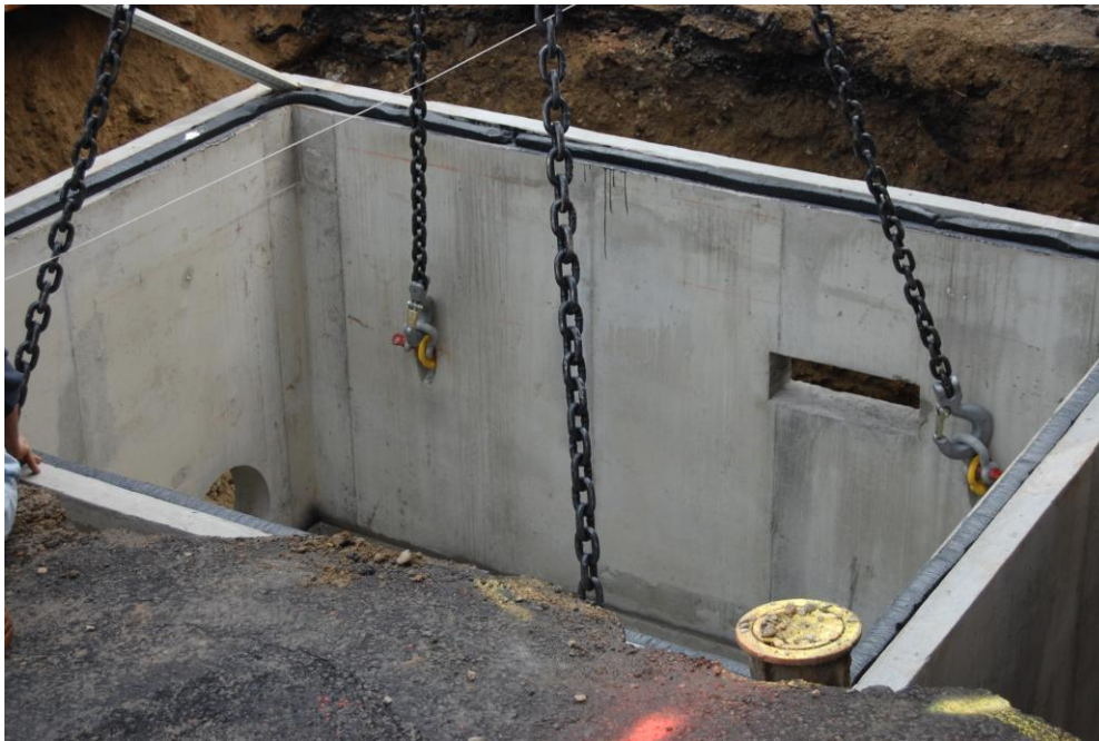
Photo 10: Note round hole for drain pipe to municipal stormdrain system and rectangular hole for tree root expansion.
