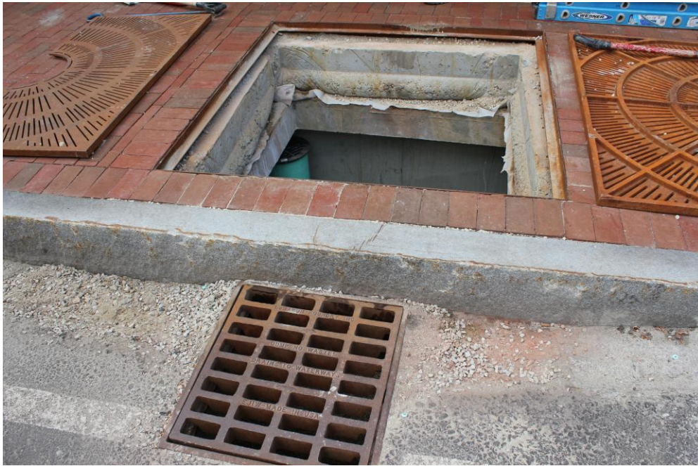
Photo 13: Note paving, curbing and brick sidewalk installed in preparation for soil and tree installation.
