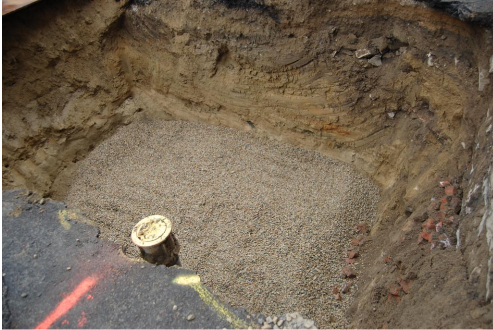
Photo 9: This is a view of the base layer of crushed stone right after installation.
