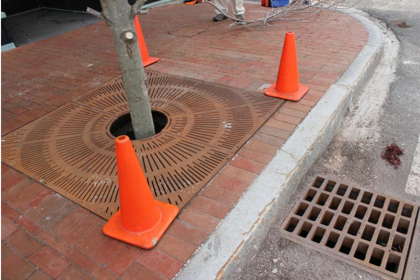
Photo 5: This is a view of the completed installation. The storm drain allows stormwater into the tree box. Sidewalk grates help prevent soil compaction. The newly installed tree had to have its lowest branches trimmed, not ideal for a newly planted street tree but necessary in this case.
