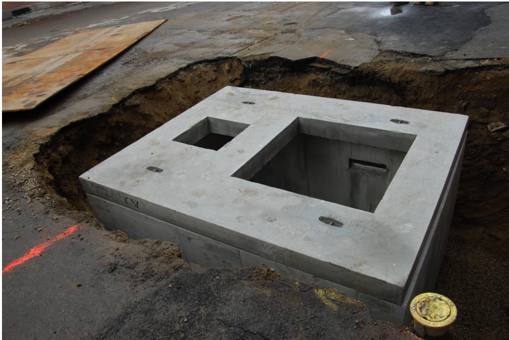
Photo 12: This is view of box and cover installed. Note cutouts in box cover for tree (larger one) and stormdrain (smaller one).
