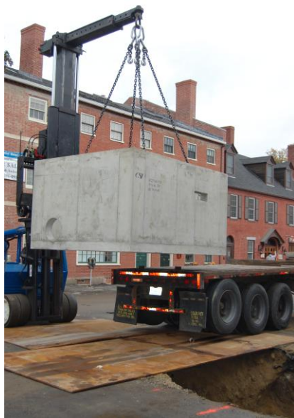
Photo 1: The concrete box is transferred from the truck to the installation site.
