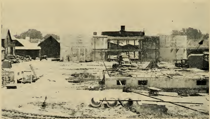
The Sludge Tanks of the Sewage Treatment plant (marked as D in the Drawing on page 52.) The pumping station foundation is in the right foreground.
