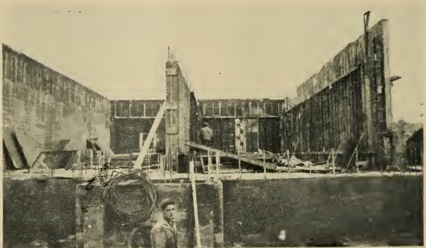
Laconia Sewage Disposal Plant showing the interior of the sedimentation tanks during construction. See page 52.
