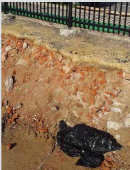
Design materials are where you find them: demolished bricks formed a permeable layer that improved the playground's stormwater performance.
