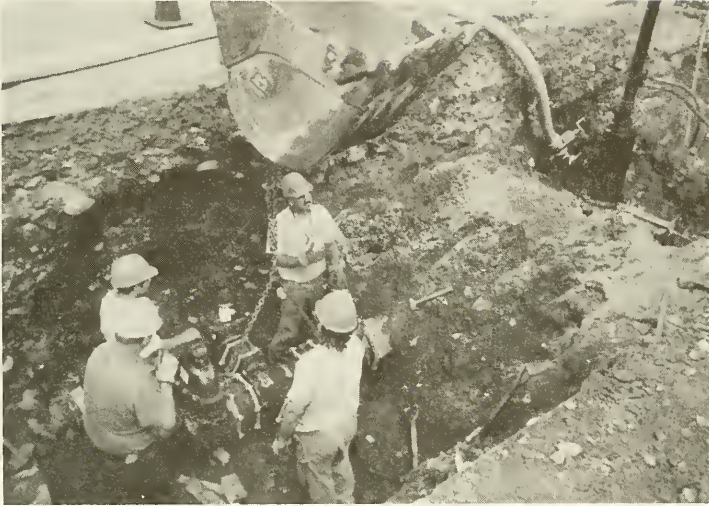
Crew readies a 12" x 8" cross and four new valves for the Main St. and Malloy St. intersection. All work was conducted without interruption of water flow.
