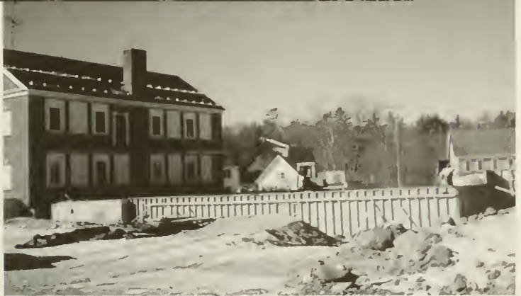
...The sounds of bulldozers and earth movers filled Bennington's air through the fall and winter of 1996-97. Pierce School's new foundations rise above the snow...five months before the first day of school '97.
