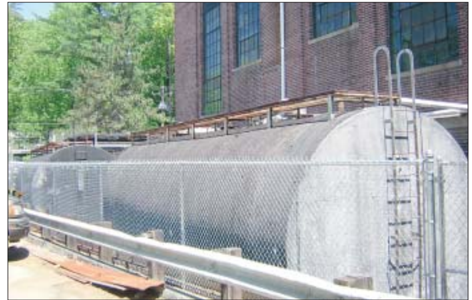
These storage tanks, located next to the UNH Central Heating Plant hold the number 6 fuel oil that is burned inside the plant to produce steam and hot water.
