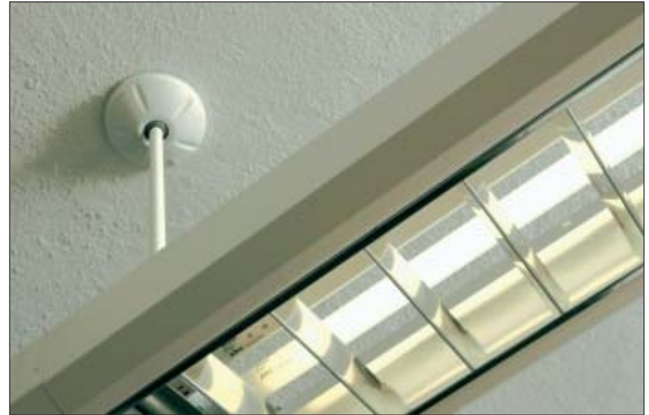
The UNH Energy Office has installed more than 30 energy efficiency projects that include lighting retrofits, heating controls, and replacement of outdated equipment. Energy efficient light fixtures (above), large windows, and glass office doors, were installed in the Nesmith Hall renovation, the home of the Office of Sustainability Programs.
