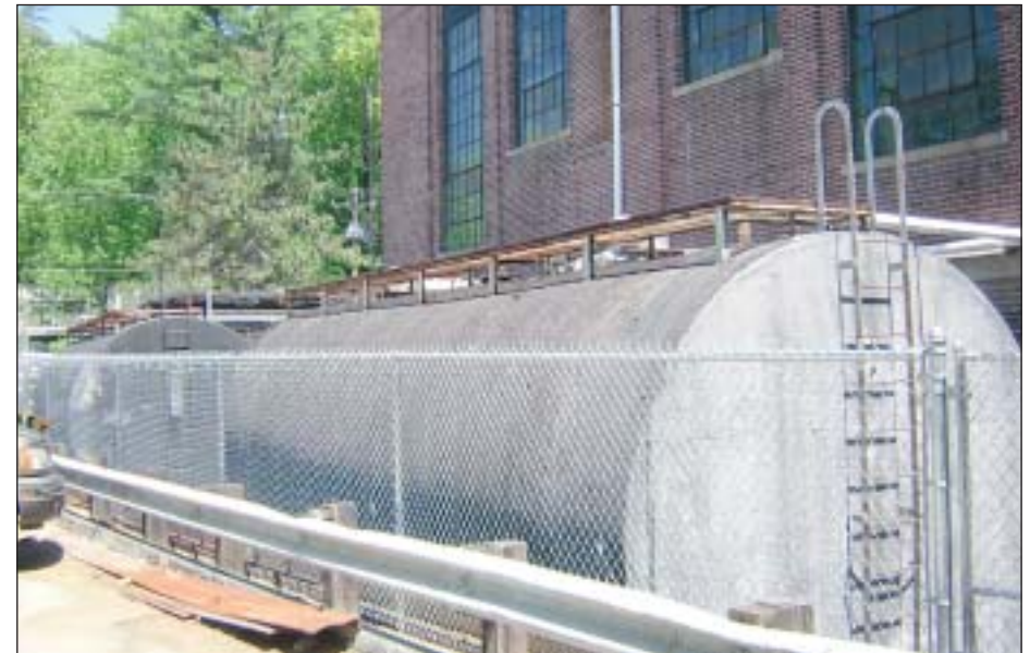
These storage tanks, located next to the UNH Central Heating Plant hold the number 6 fuel oil that is burned inside the plant to produce steam and hot water.
