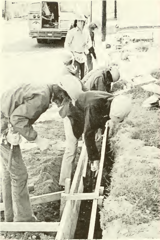
Vocational Education Program Students working "on job" laying curbing for side walks.
