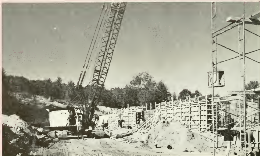
A concrete placement is under way on one of the wall sections for the aerator tank, located just to the north of the operations bldg.
